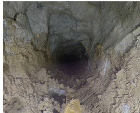
(b) Poor condition
