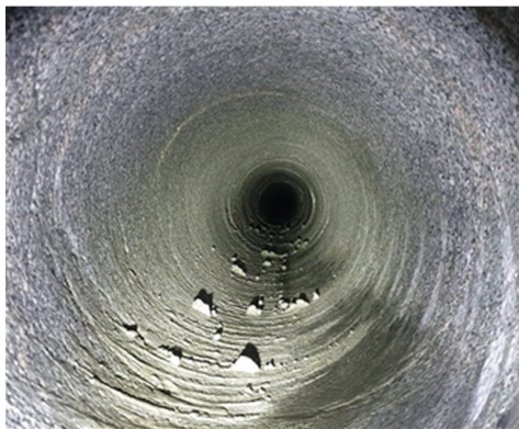
(a) Good condition
